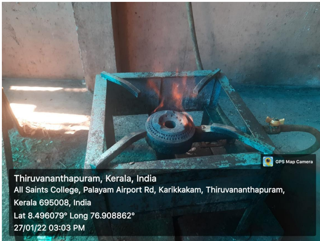
BIOGAS PLANT AND BURNER AT THE ALL SAINTS' COLLEGE CANTEEN
