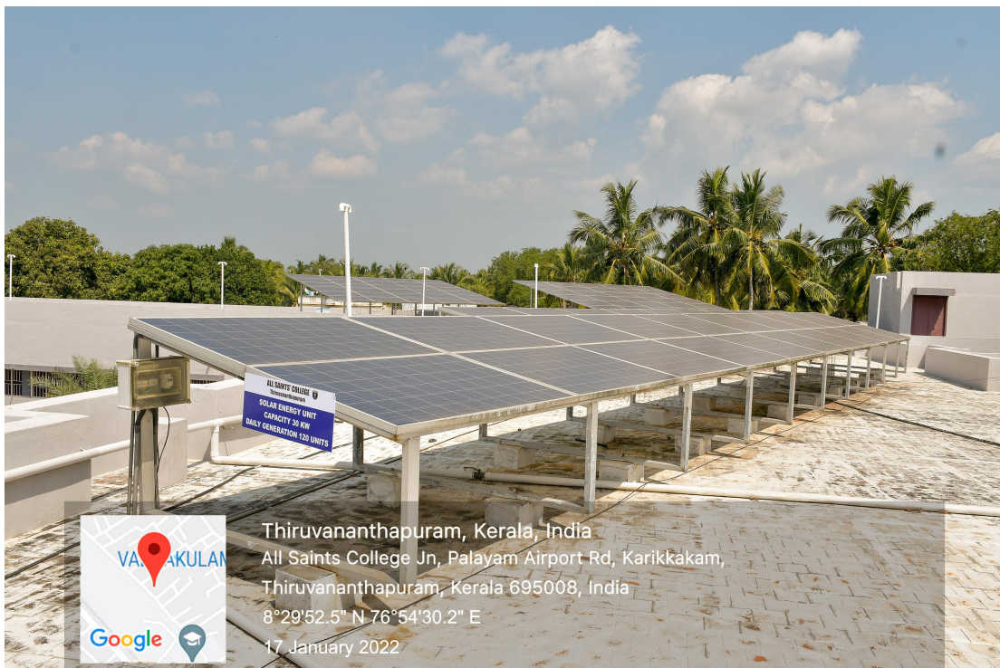
SOLAR ENERGY FACILITY-1 IN THE CAMPUS WITH A CAPACITY OF 30 KW WITH DAILY GENERATION OF 120 UNITS
