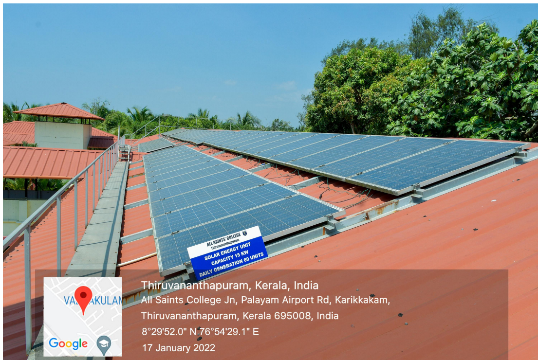
SOLAR ENERGY FACILITY-2 IN THE CAMPUS WITH A CAPACITY OF 15 KW WITH DAILY GENERATION OF 60 UNITS
